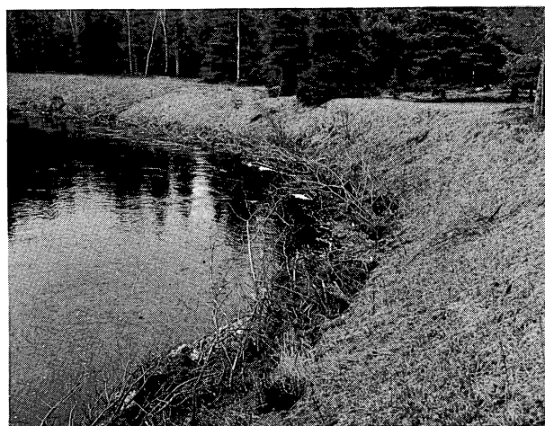
F-517760 FIGURE 11. — A bank stabilized with whole trees. This structure will need continual maintenance.
