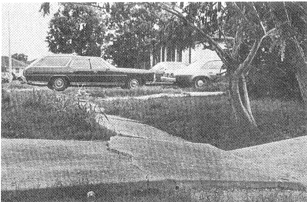
Figure 10.—Warped and cracked sidewalk on corner of E. Lemans and Dwyer Streets, Village Del-Est subdivision, New Orleans.
