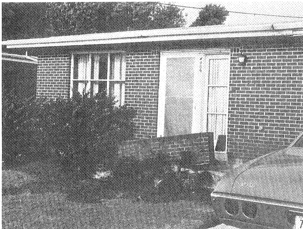
Figure 11.—Residence at 4309 Williams Boulevard, Kenner, with advanced tilting and cracking of low brick wall.
