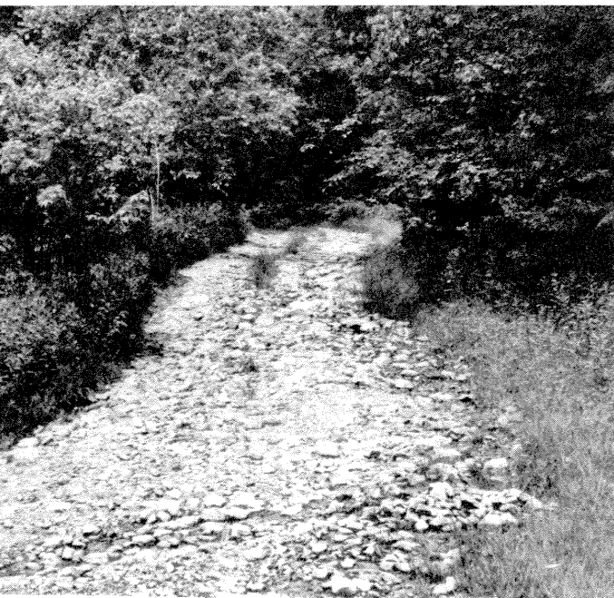
Figure 17.—Erosion pavement on a logging road with an 8-percent grade near Canyon Rim Road, Blackwater Falls Park. This was the most severely eroded road found and most of the soil loss probably occurred before the storm of May 24.
