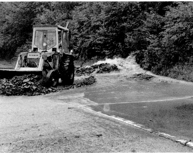
Figure 2.—Highway workers were pressed to keep Route 38 open to traffic as debris poured from this unnamed draw near St. George. At this elevation (1,700 feet) tree foliage had almost fully emerged.
