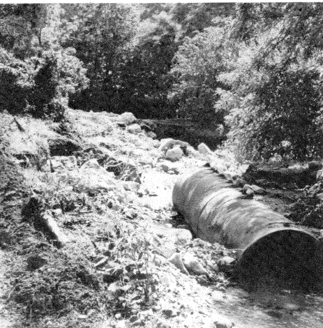
Figure 24.— This 4-foot culvert had provided access to a small farm on the right. Dumplin' Run washed away the newly repaired gravel road on the left.
