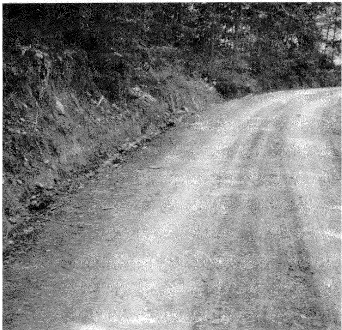
Figure 22. —These road banks are 8 feet high, the ditches 2 feet deep, the traveled road surface 24 feet wide. The roadbed is on sandstone bedrock at a grade of 9 percent. The road was completely washed out by the flash flood.
