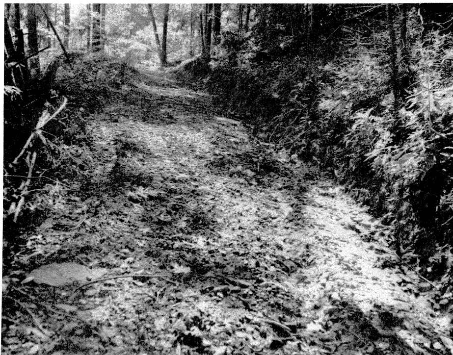
Figure 9.—This road suffered little or no erosion even though it was insloped and on a 15 percent grade.
