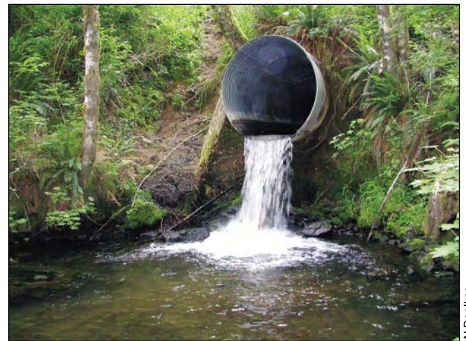
Figure 54—Culverts with steep drops at the outlet can be barriers to upstream fish passage.
