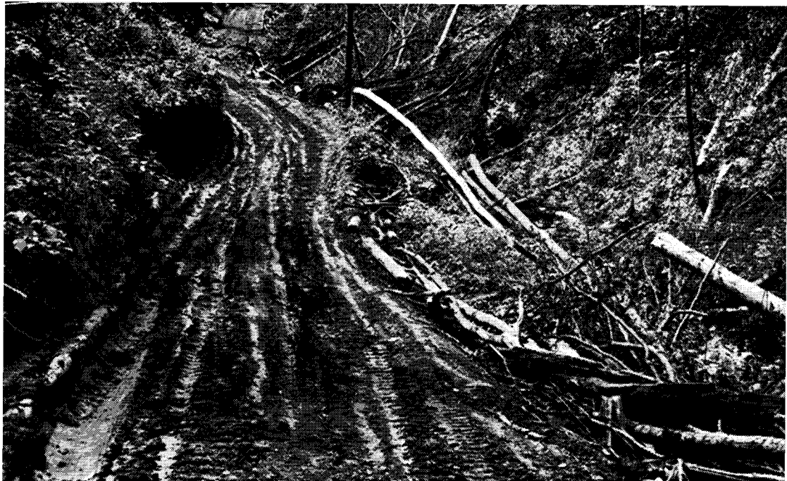
Figure 9.—Serious stream pollution occurred when this logging road was located too close to a stream. The filter strip between the road and stream was not wide enough to prevent mud washed off the road from reaching the stream.
