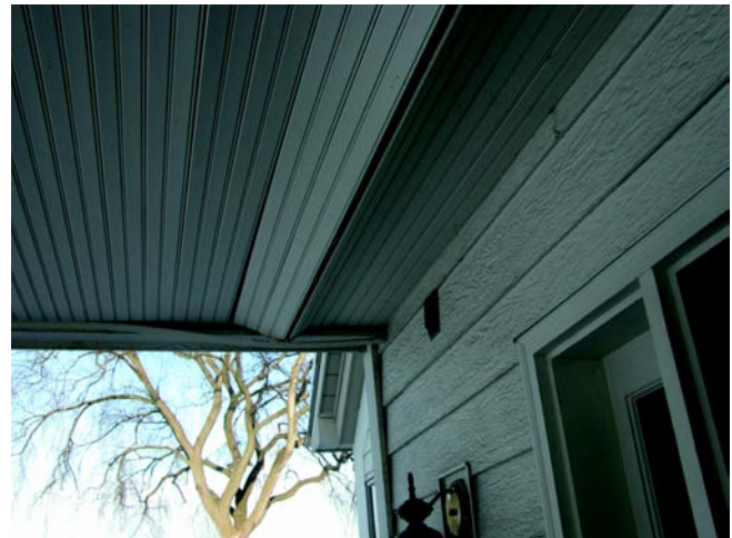
Figure 4 Buckled flat-grain pine pattern lumber on porch ceiling in late December of 2005. In contrast to lumber on ceiling, OSB lap siding on adjacent wall is not buckled. Buckled lumber is not defaced by mold or mildew.
