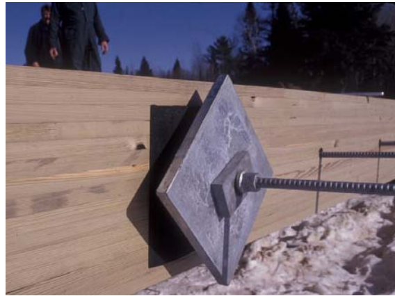
FIGURE 2 ROOF SHINGLE MATERIAL SEPARATING A STEEL BEARING PLATE FROM CCA- TREATED WOOD DECK.
