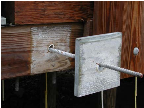
FIGURE 1 PVC TUBING SEPARATING ACQ TREATMENT FROM GALVANIZED HIGH-STRENGTH STEEL BARS WITHIN A STRESS-LAMINATED DECK DECK. NOTICE THE WHITE CORROSION PRODUCTS.
