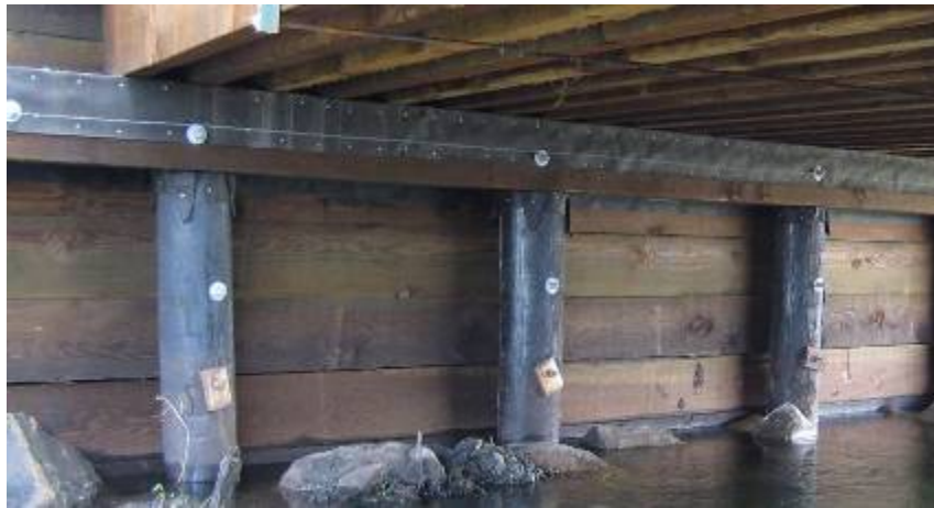
Figure 4-47. Good copper naphthenate backwall
