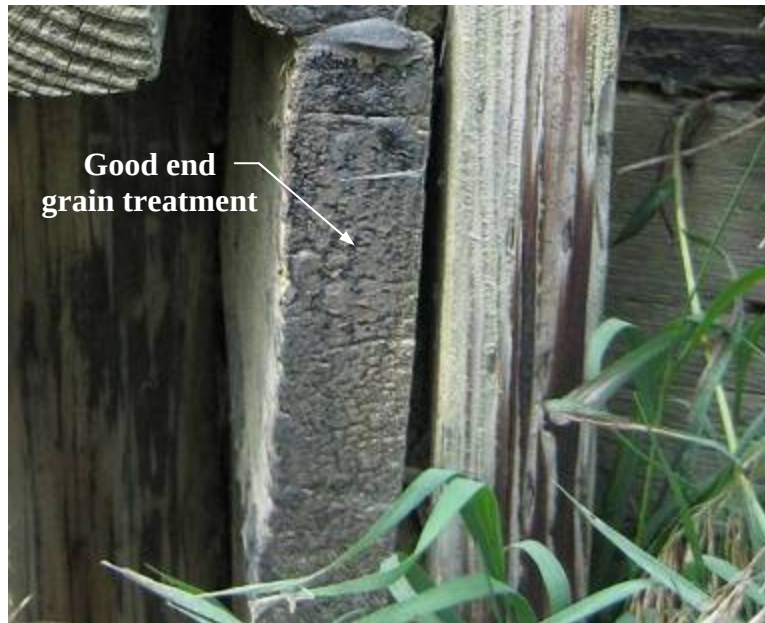
Figure 4-14. Good backwall with treated end grain
