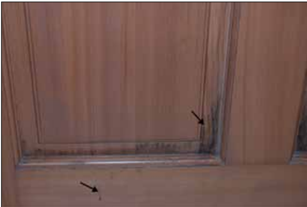
Figure 4—Mold growth on the edges of panels of the front entry door. Evidence of run-down of condensate (seen as staining and mold growth) is also apparent on the rail below the panel, particularly on the profiled edge of the rail. (Photo by Robert Munson, Forest Products Laboratory, January 10, 2008.)
