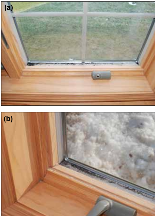
Figure 3 (a, b)—Mold growth on interior surfaces of lower rails of two representative vinyl clad window sash. Mold growth is most prevalent near pane edges and at corners, where condensate has collected. (Photo by Robert Munson, Forest Products Laboratory, January 10, 2008.)
