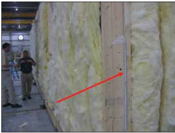
Figure A6. Corner of module showing drywall coming to end of wall section (see arrow).
