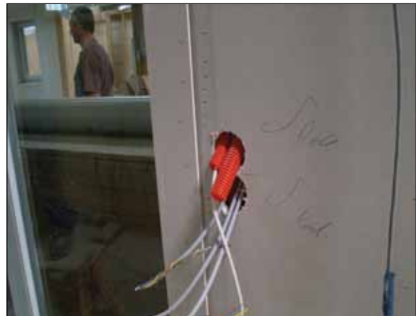
Figure GA16. Wiring conduits exiting wall panel with wiring.
