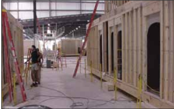
Figure F1. Looking down the “shotgun” manufacturing line toward the cross-over area.
