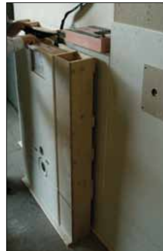
Figure GH6. Wet wall used for toilet contains installed plumbing.
