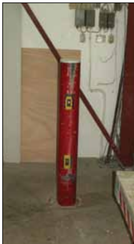
Figure GC7. Light curtain reflector at wall table used to protect workers during clamping by halting clamping operations if workers break the light perimeter.
