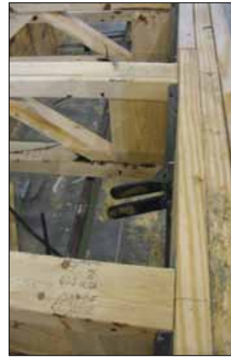
Figure B3. Open Joist 2000 floor joists were used but could not fit into the positioning fingers shown.
