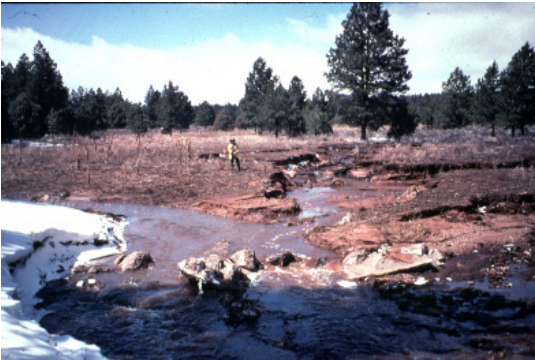
Figure 5 —Major erosion due to spring 1998 flooding. This photo is taken looking upstream from the fenceline project boundary. The second to last constructed concrete weir is in the center of the photograph.
