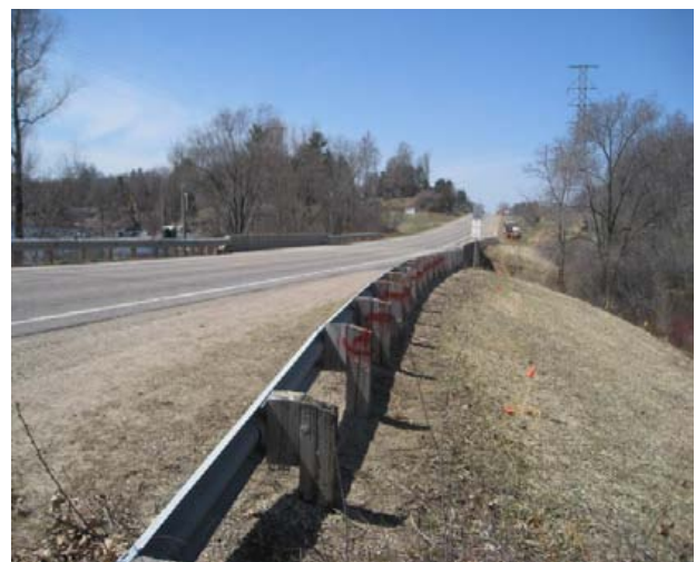
Figure 9: Merrimac field site showing old posts in-service
