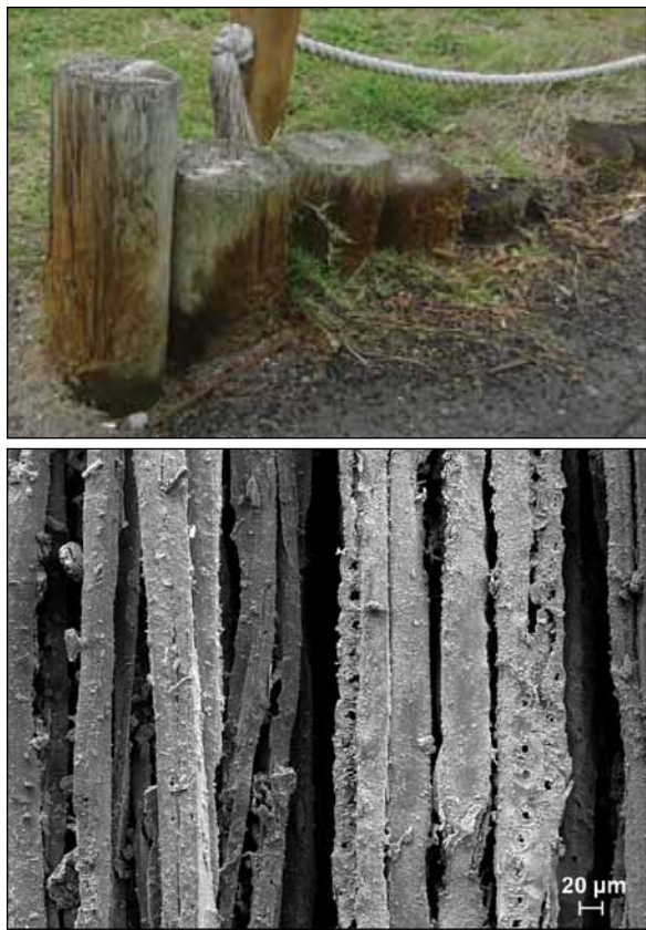
Figure 2. Image of salt-damaged pilings and corresponding sample showing tracheid separations and no fungal presence using SEM (175× magnification).
