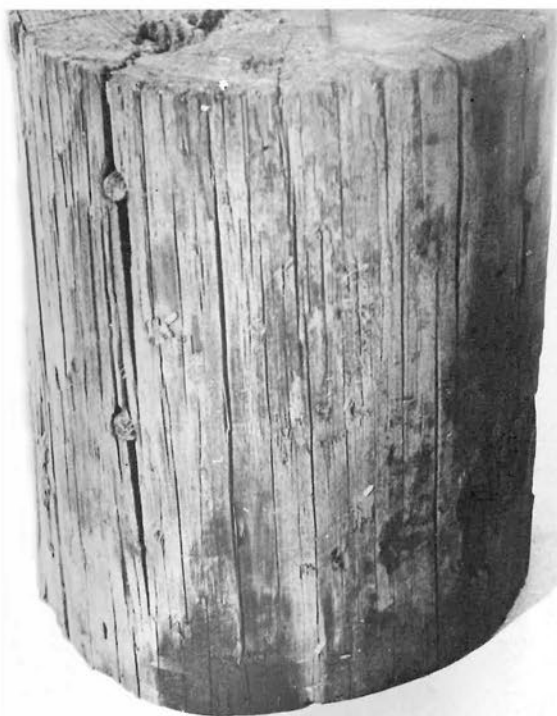
Figure 30.—Decay associated with deep checks initiated by increment borer holes plugged with wood dowels.
