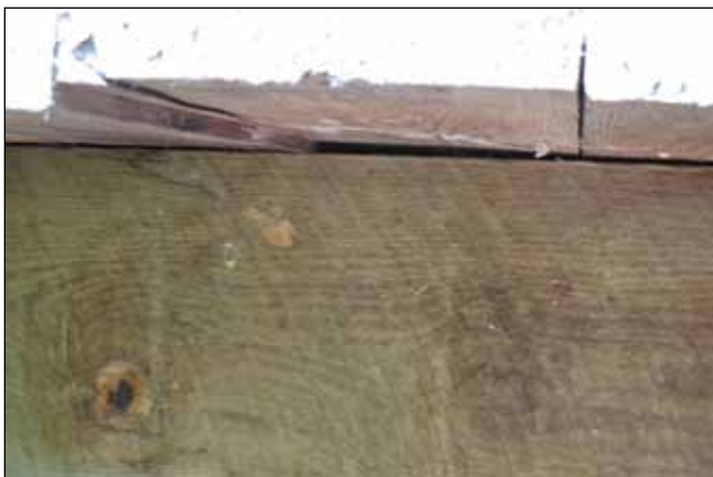
Figure F15. Deck board detachment.
