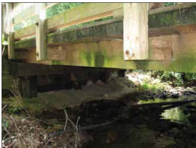
Figure J14. Moss growth on girder 19.
