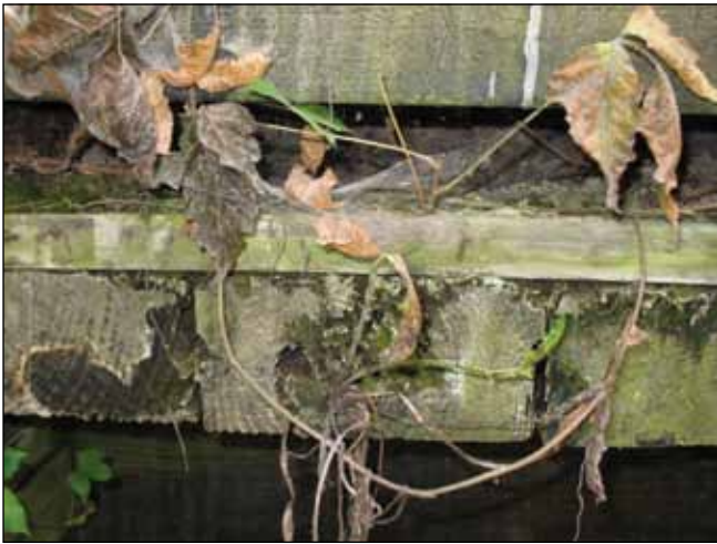
Figure I13. Decay in the ends of the deck boards.
