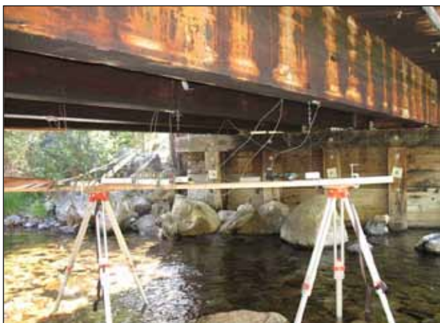
Figure Q6. Deflection instrumentation.
