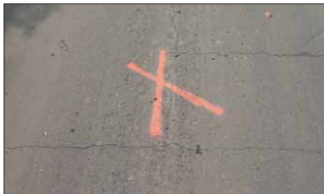
Figure D13. Pavement chipping at west end.
