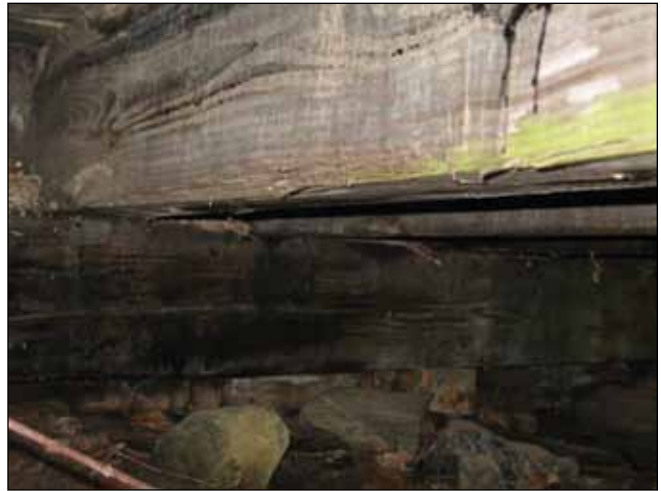
Figure I16. Mechanical damage to girder.
