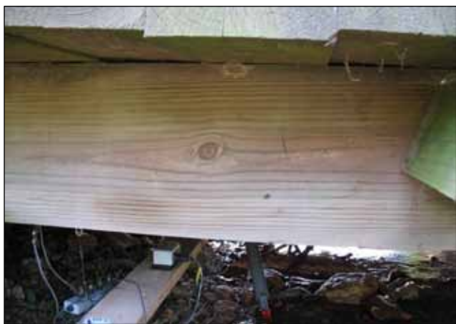
Figure E14. Deck board detachment.
