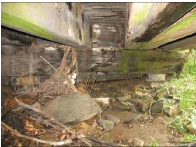
Figure I15. Fungal growth throughout superstructure.
