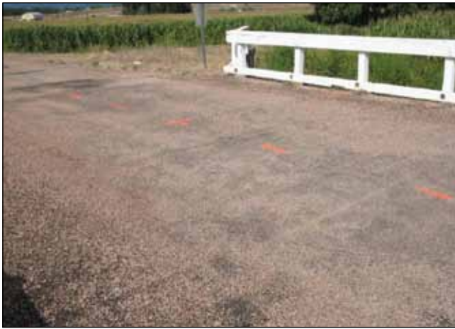
Figure K13. Transverse wearing surface cracking.
