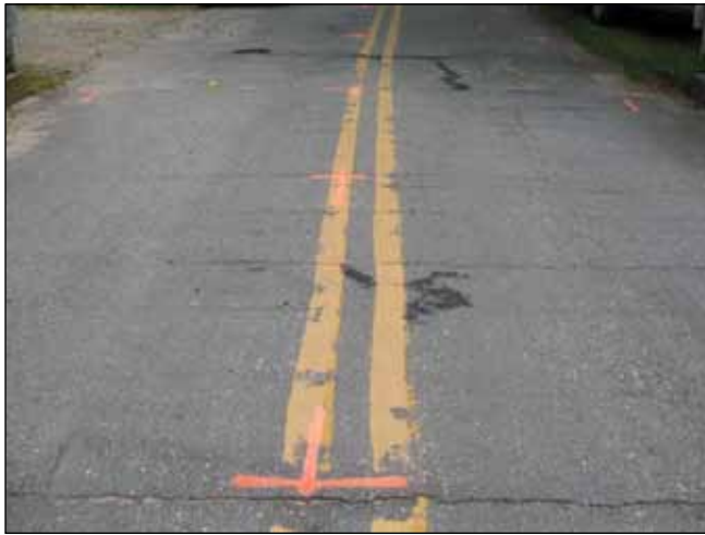
Figure F13. Presence of transverse cracks.
