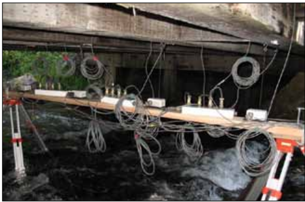
Figure P6. Deflection instrumentation.
