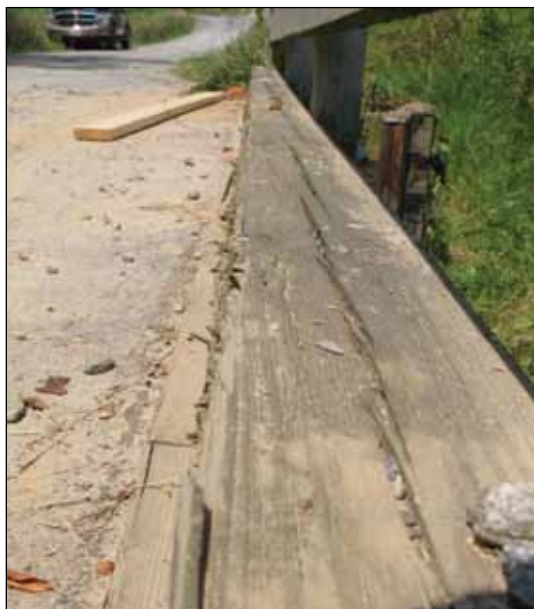
Figure H15. Advanced degradation throughout curbs.
