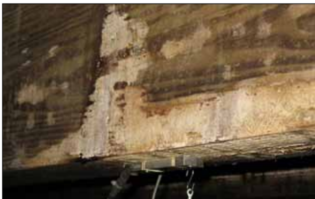
Figure C14. Biotic growth on girders.
