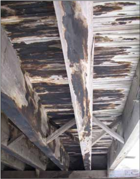
Figure O13. White residue formation on deck.
