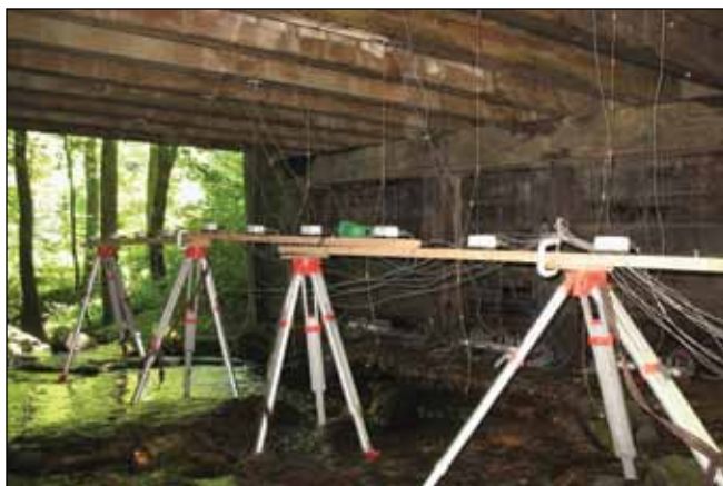
Figure 4. Typical deflection gage instrumentation.
