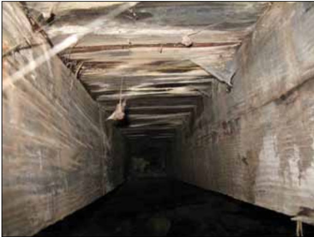
Figure I14. Girder and deck condition.
