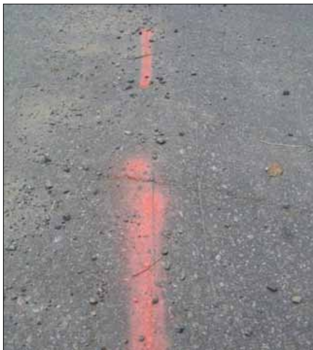
Figure H13. Minor transverse cracks.
