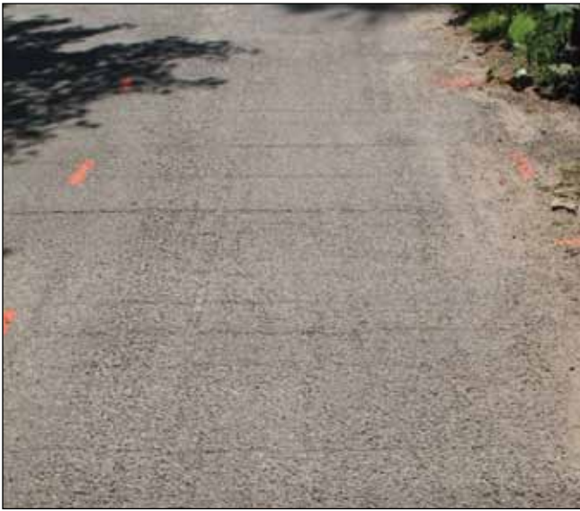
Figure G13. Transverse cracks in the wearing surface.
