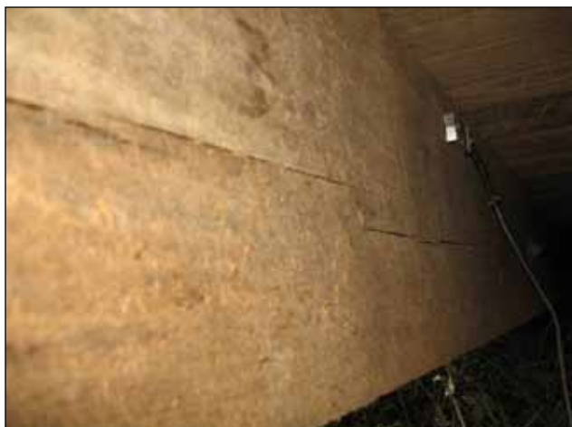
Figure E15. Observed checking in girders.
