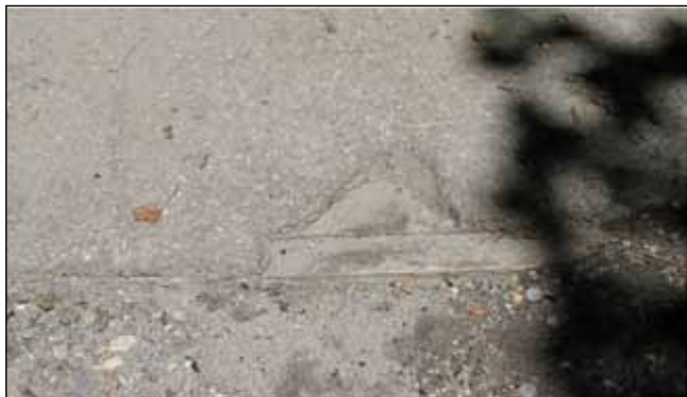
Figure C13. Pavement chipping at west end.
