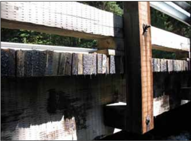
Figure P14. Twisting of deck boards.
