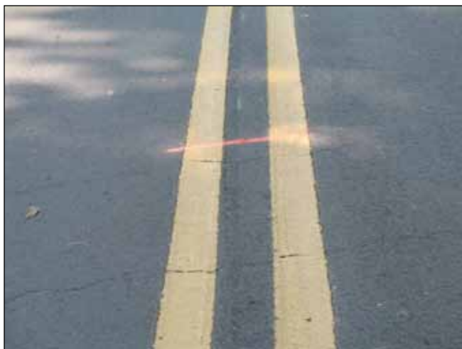
Figure J13. Observed transverse cracks.
