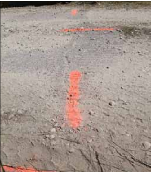
Figure Q13. Wearing surface cracking and debris.
