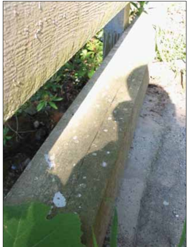
Figure G16. Parapet condition.
