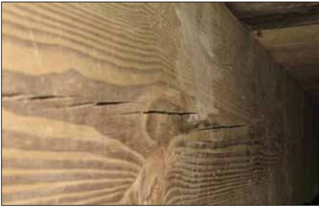
Figure D15. Checking at centerline of girder.
