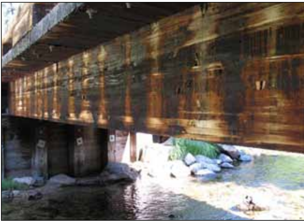
Figure Q15. Girder streaking and holes.
