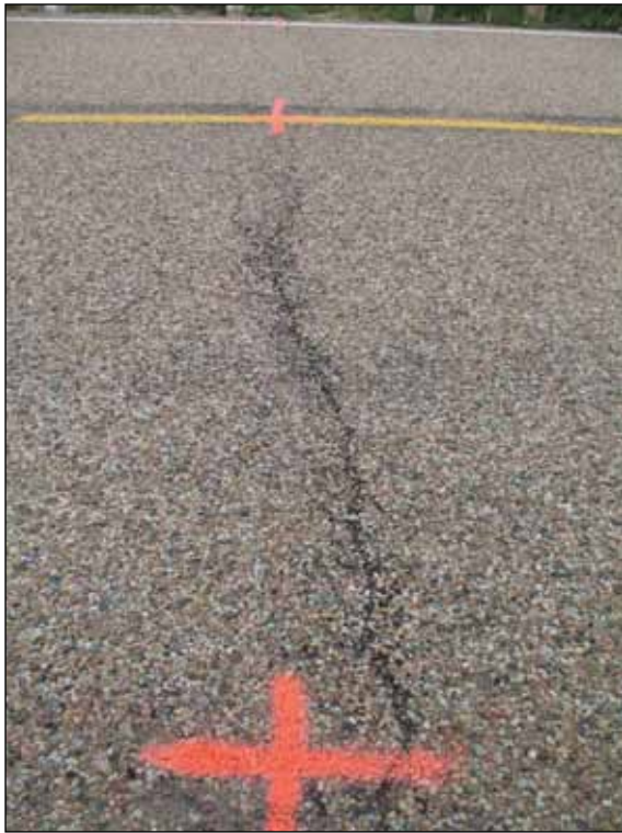
Figure L13. Transverse wearing surface cracking.
