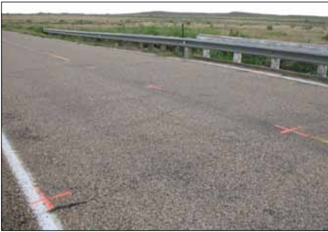
Figure M13. Transverse wearing surface cracking.
