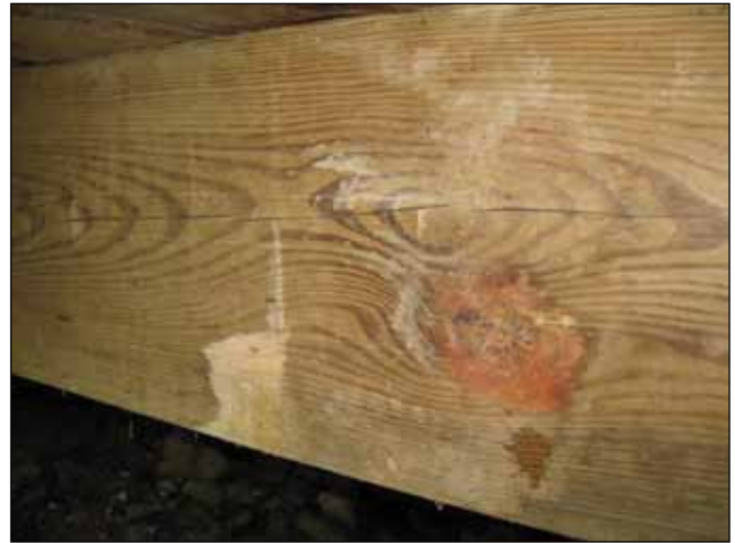
Figure F16. Checking at girder centerline.
