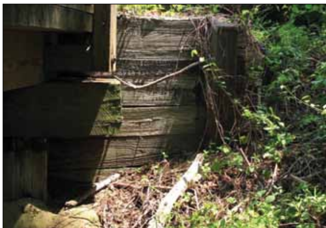
Figure J15. Wingwall weathering and decay.
