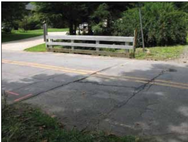
Figure F14. Transverse cracks at bridge approach.
