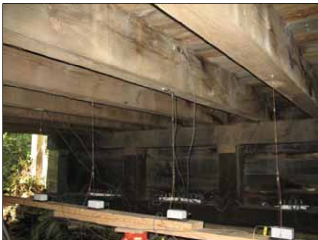
Figure G6. Deflection instrumentation.
