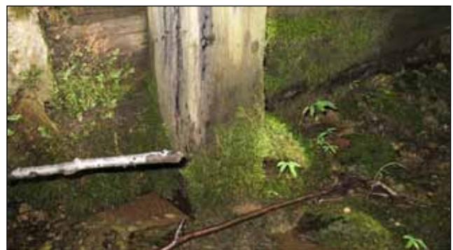
Figure C15. Moss growth at base of substructure posts.
