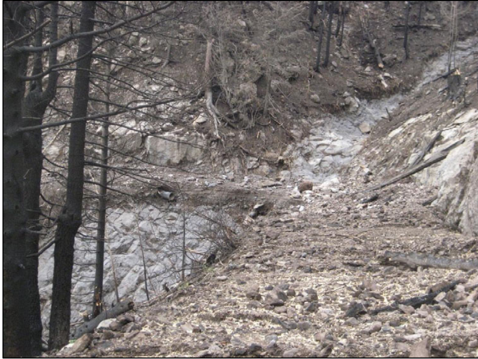
Figure 9. Photo taken on July 25th of FR146 at the drainage where the waterline was severed and removed by debris flows on July 20th. Half of the roadbed was removed by the debris flows; the remaining roadbed was removed during the August 16th debris flows. Photo: D. Fleishman, USFS.
