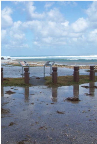
Damage at War in the Pacific National Historical Park from 2002's Typhoon Pongsona; NPS photos.
