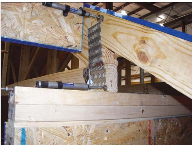
Figure 14. Truss member displacement and metal connector plate deformation at heel joint (Specimen A).
