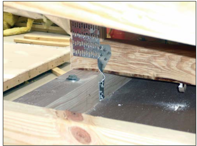
Figure 15. Buckling of hurricane clip (Specimen C).
