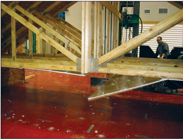
Figure 12. Complete failure of gypsum fasteners (Specimen A).
