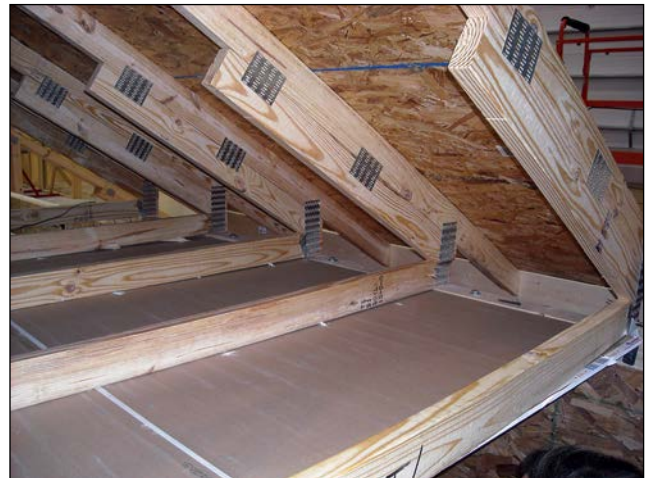
Figure 11. Gypsum fastener tear-through (Specimen A).
