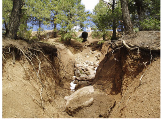
Figure 4. A gully formed at a culvert outlet. Gullies in the study area are developing in the downslope direction. Source: Troendle et al. , unpublished report. 2010, pp 1–34. This figure is available in colour online at wileyonlinelibrary.com/journal/espl
