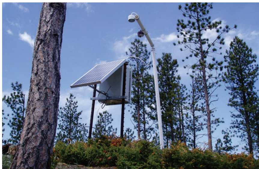
Figure 3 —Version 3.1 installation on the Black Hills National Forest showing inlet support, instrument/battery enclosure and 40W solar panel.
