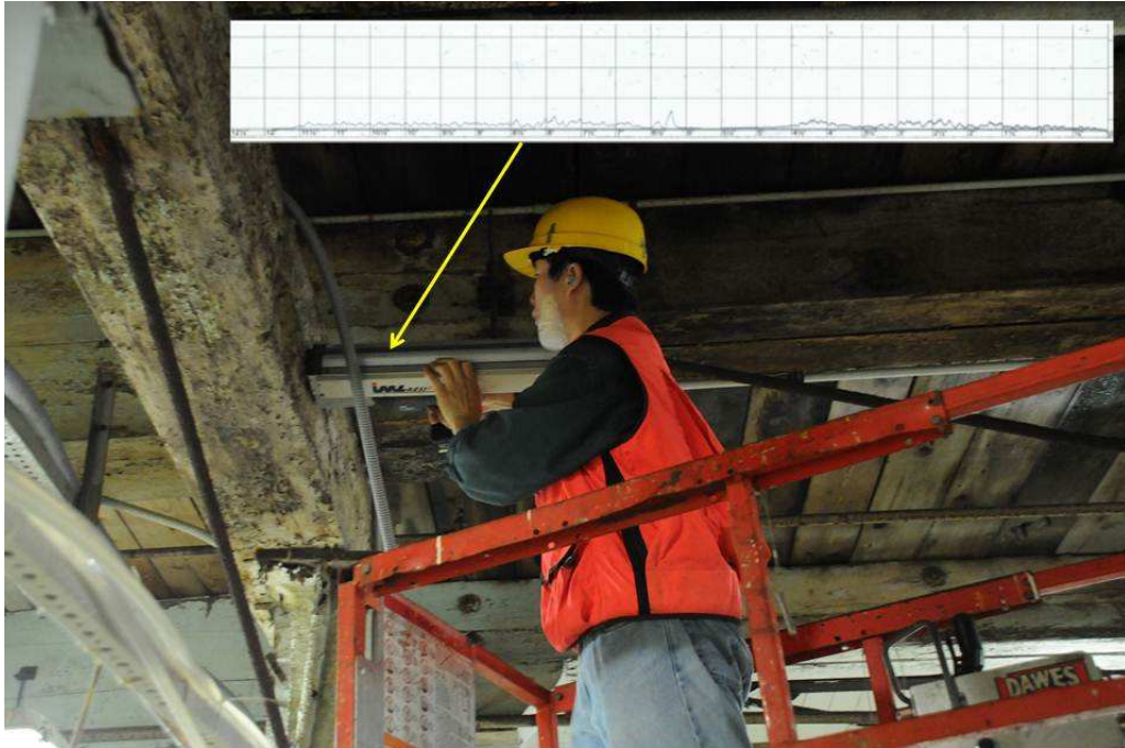
Figure 6. Longitudinal beam in row A: resistance drilling test showed little or no resistance, an indication of severe internal rot.
