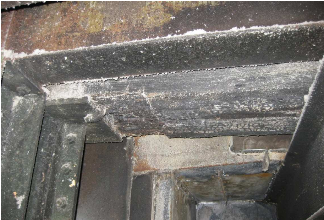
Figure 7. Longitudinal beam between A8 and A9a exhibits fire damage. The effective cross-section of the charred beam has been reduced significantly.
