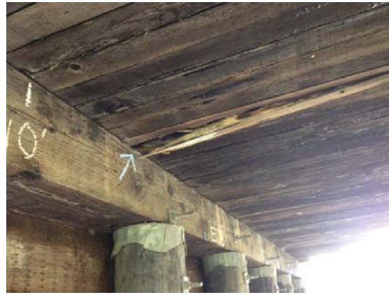
Fig. 13 Damage at longitudinal deck panel connection, Clarke 3
