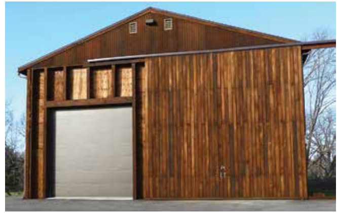
Figure 9. Oil-based copper naphthenate is sometimes used for treatment of salt storage sheds.
