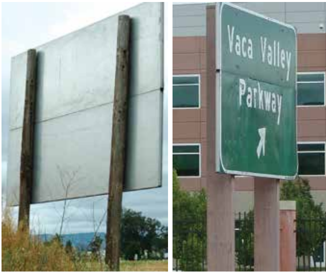
Figure 27. California uses round poles or large sawn posts to support larger highway signs.
