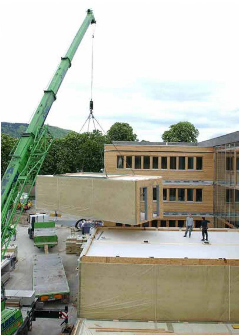
Figure 24 Impulsezentrum, Graz, Austria (courtesy of KLH)
