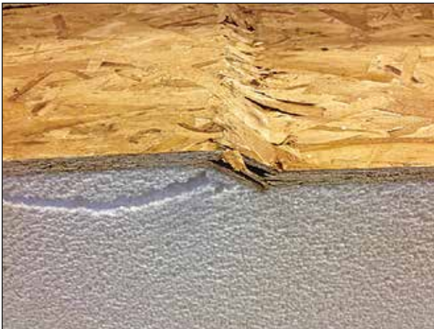
Figure 13. Compression failure (FPL).
