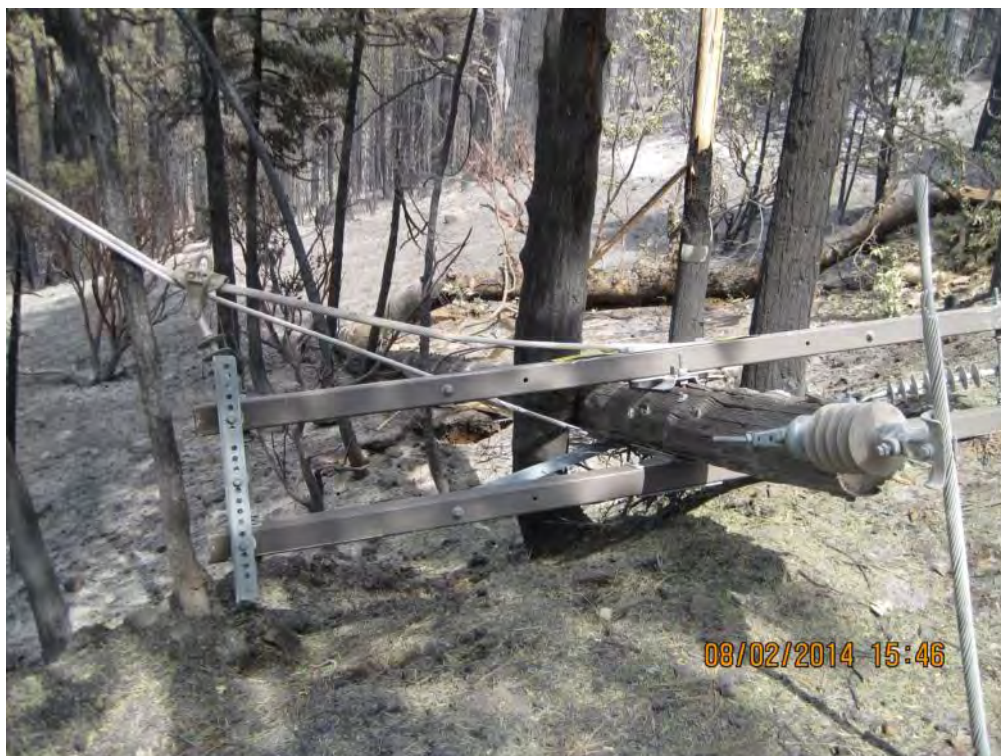
Photo: A downed power transmission pole and line on the French Fire in California in 2014. Photo courtesy of Bret Butler / FFS.
