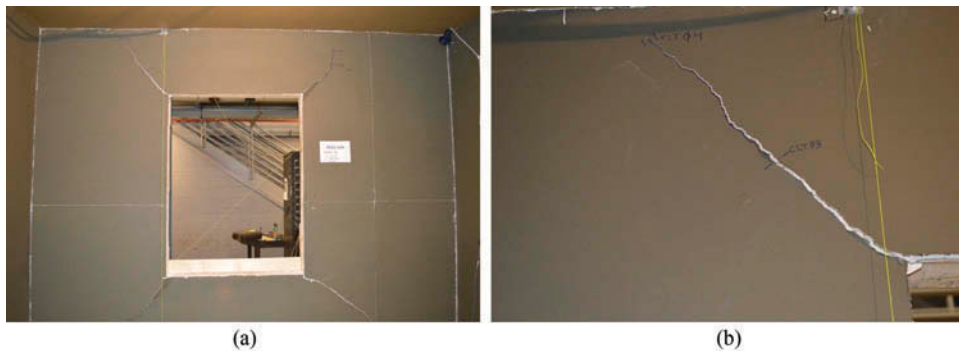
FIGURE 13 Damage caused during CLT retrofit test program on second story south wall: (a) damaged GWB and (b) close-up of top left window corner.
