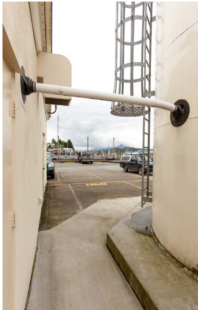
Pellets are transported from the exterior pellet silo (right) into the boiler room (right) through this 4-inch flexible auger.
