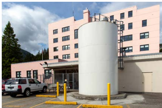
The white external 20-ton silo holds enough pellets for several months of heating.
