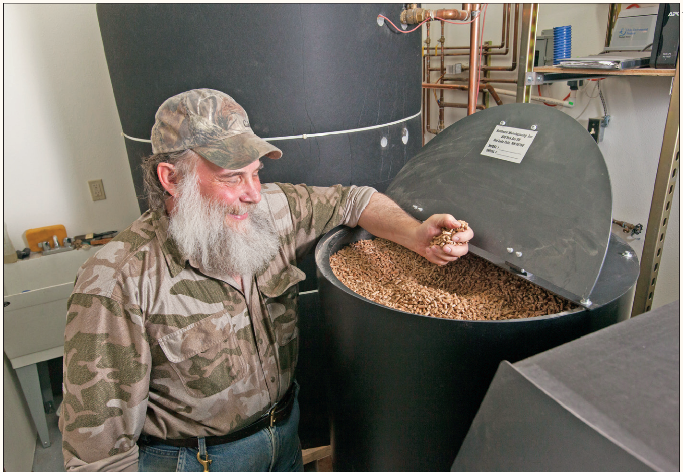
Jim Baichtal shows the wood pellet boiler that heats his home in Thorne Bay on Prince of Wales Island. A Forest Service study found that the biggest factor in Alaskan homeowners' willingness to convert to wood energy came down to the financial trade-off between the cost of heating oil and the investment needed to switch to a wood-burning appliance.
