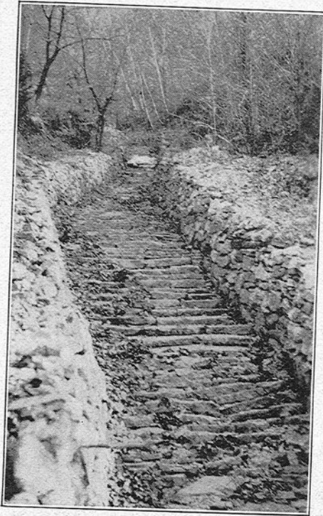
FIG. 58.—ROCK-LINED CHANNEL BUILT NEAR FOUNTAIN CITY, WISCONSIN
