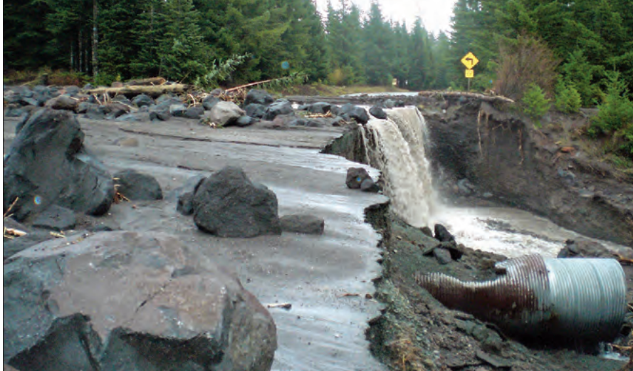
Flooding and subsequent damage to roads and infrastructure, like this may become more common as winter precipitation shifts from snow to rain. Above, a washout on the Gifford Pinchot National Forest.
