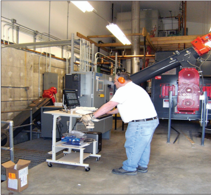
Figure 11—Boiler control system.
