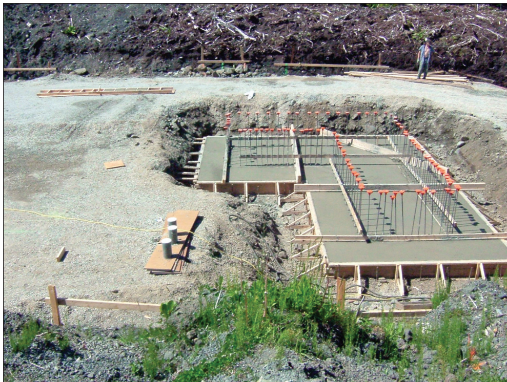
Figure 7—Concrete foundation of the Craig boiler system.
