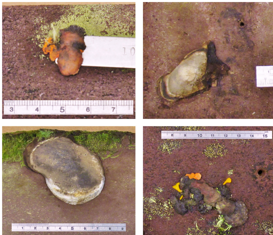
Figure 4. Examples of decay fungi fruiting bodies observed after 8 years of exterior exposure.
