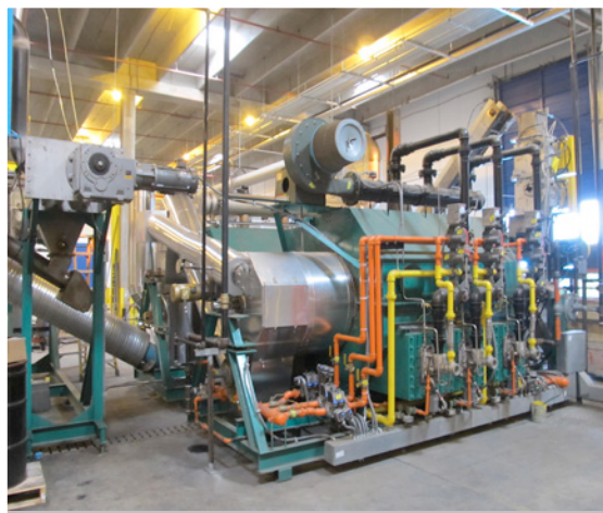
The Tucker RNG thermal conversion system deployed at ReVenture Park, Charlotte, NC.
