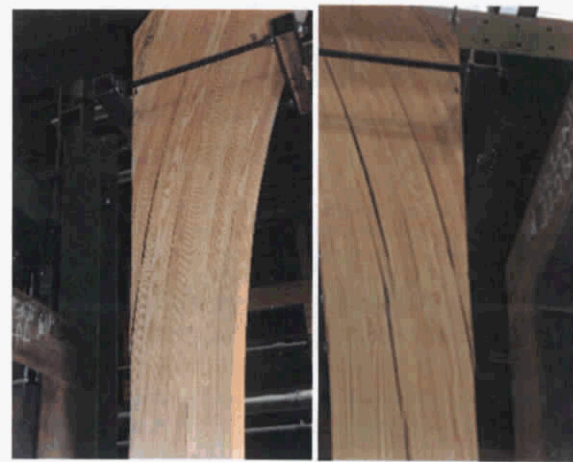
Figure 9: Radial tension failure for first tested arch
