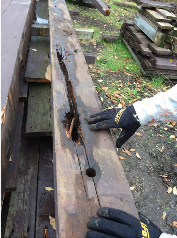
Figure 12. Horizontal support member that contained severe deterioration.
