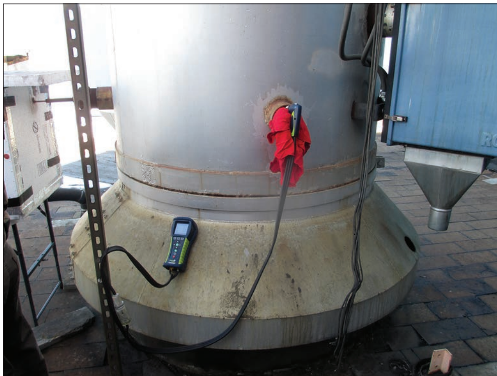
Figure 9—Bacharach PCA3 probe inserted into combustion flue gas stack (with red cloth, center); Testo probe inserted into the stack at the left side of photo.
