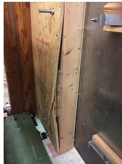
Figure 12. Damage caused by impact adjacent to door opening. No debris created, but deflection >3 in. occurred.
