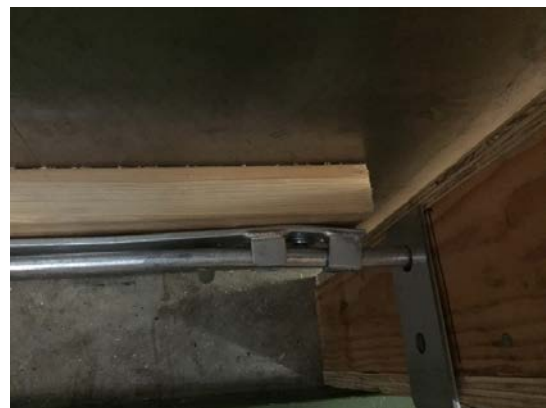
Figure 28. Bending of cane bolt caused by wind suction at two times design load.
