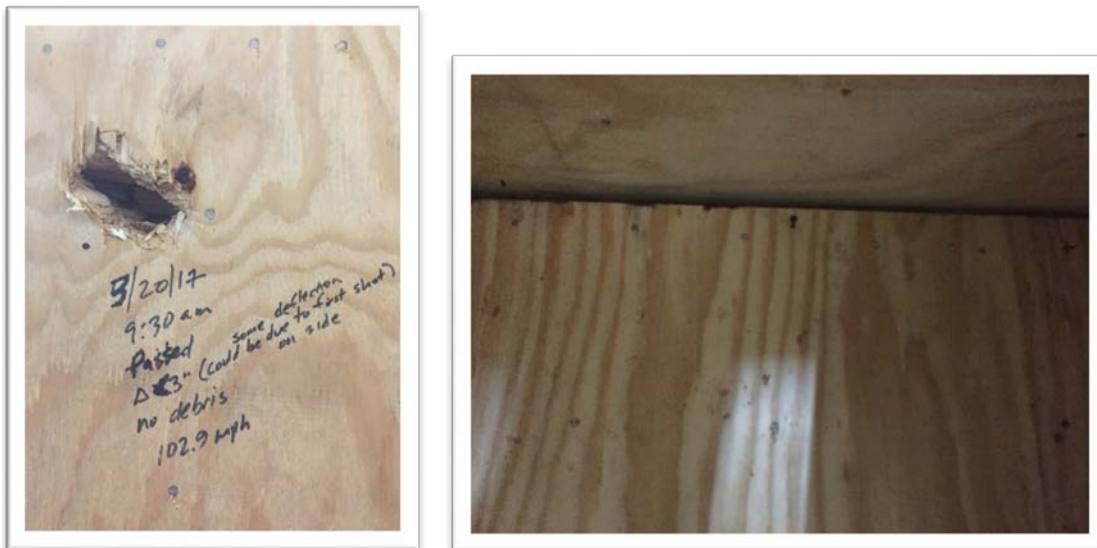
Left: exterior damage after impact; Right: interior damage after impact. (impact location: 27 in. left of center, 8.5 in. below top of room side.)
