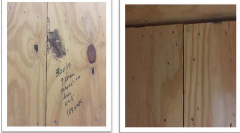
Left: exterior damage after impact; Right: interior damage after impact. (impact location: 1.5 in. right, 7.5 in. below top center of room side.)
