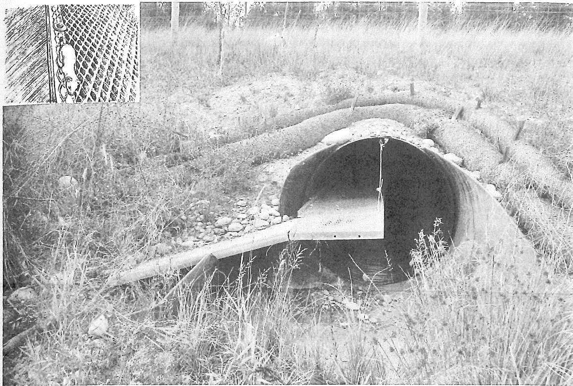
Figure 10.1. Installation of a bolt-on metal shelf, produced by Critter-Crossing Technology, LLC, for small animal passage within a drainage culvert, as shown by drawing (based on an actual image) of a short-tailed weasel ( Mustela erminea ) crossing the shelf (inset). Credits: Reproduced by permission of Kerry R. Foresman; © Victor Young Illustration (inset, adapted from original photo by Kerry R. Foresman).
