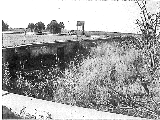
Figure 10.5. The Paynes Prairie wall and culvert passage system, Florida, United States. Credit: Daniel J. Smith.
