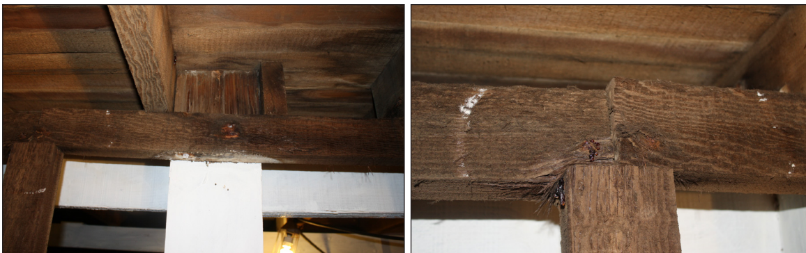
Figure 3. (Left) New structural members to hold up deck; (Right) Structural failure of old wooden beams caused by salt damage.
