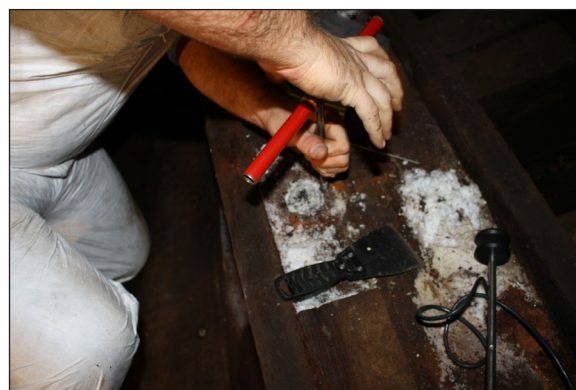
Figure 6. Increment core being taken on a keelson near two corroded bolts that were identifiable by white corrosion product blossoms.
