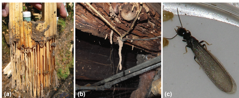
Figure 4. (a) Termite damage to Southern Pine; (b) shelter/mud tubes; (c) alate.
