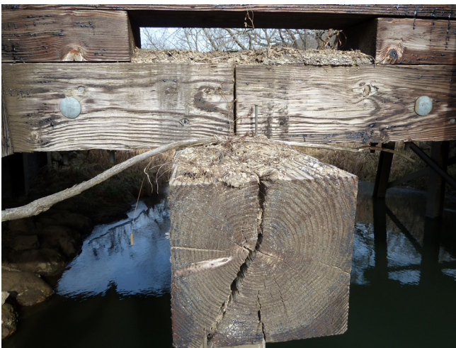
Figure 3. Drying checks in bridge timber.
