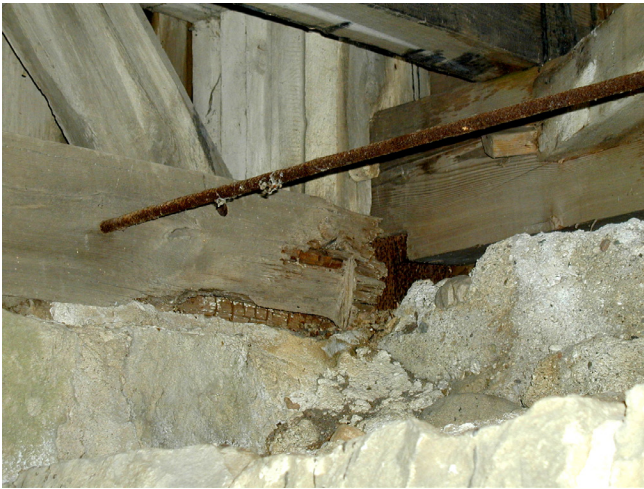
Figure 2. Area in covered bridge members that often exhibit problems with moisture where they come in contact with an abutment or supports at the ends of the bridge.
