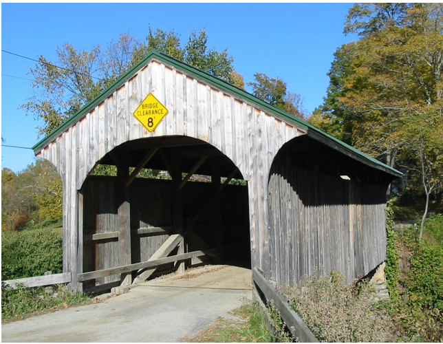
Figure 1. Members at ends of covered bridge are vulnerable to wetting from wind-blown rain because of the very small overhang.
