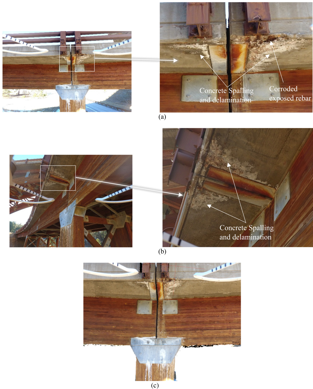
Fig. 9. Underside of deck sample damage gathered using drone (taken by Junwon Seo): (a) concrete spalling and corrosion with exposed rebar near Girder 4 at Joint 1; (b) concrete spalling near Girder 4 at Joint 3; and (c) 3D virtual model of Joint 2 near Girder 4 using PhotoScan.
