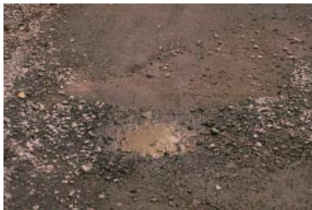
Figure 19—Soil on deck surface should be removed, and potholes along end of bridge should be filled.
