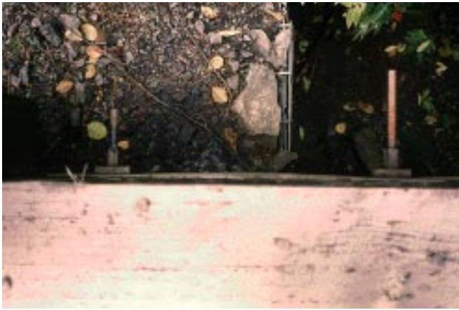
Figure 20—Crushing of outside laminations, causing a wave distortion of the bearing plates.
