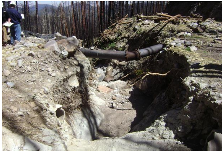
Figure 31. Damaged water pipeline after the 2010 Schultz Fire, Coconino National Forest, Arizona (Photo courtesy of the City of Flagstaff, Public Works Department).
