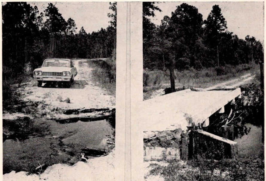
FIGURE 1.—Forest roads over-topped and under-mined by flood waters from coastal forests.
