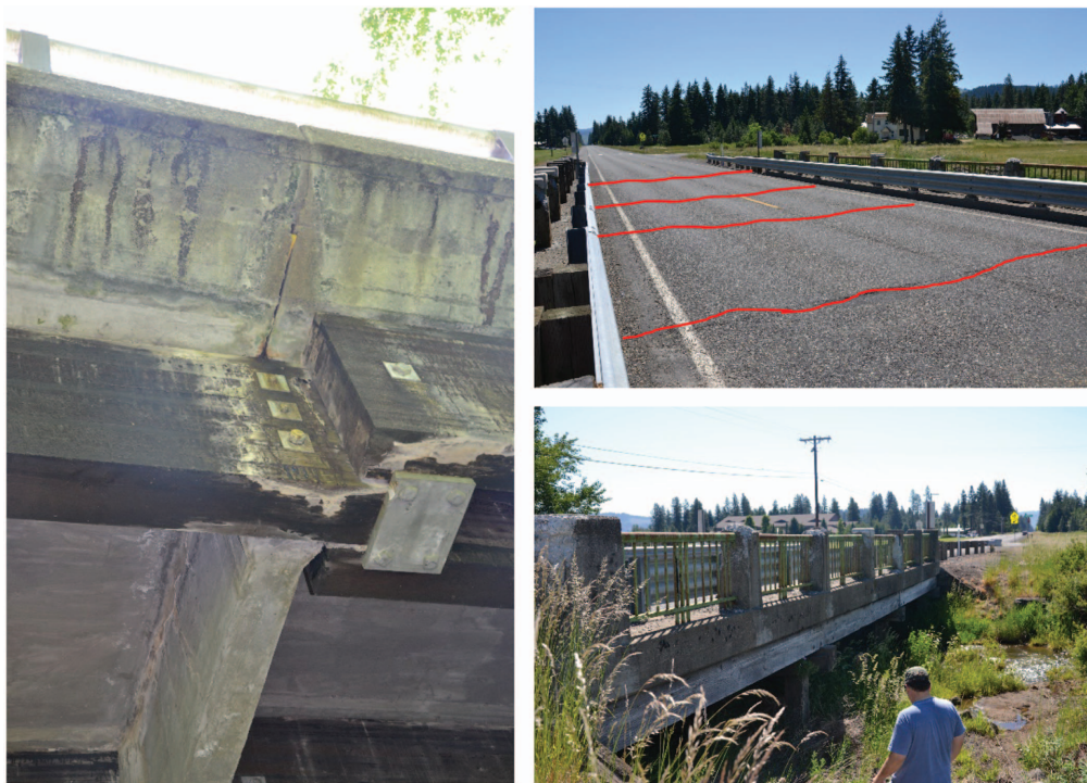
Fig. 12. (Color) Expansion joints and crack in the concrete member allowing water into the glulam girders. (Images by Alfredo M. P. G. Dias.)
