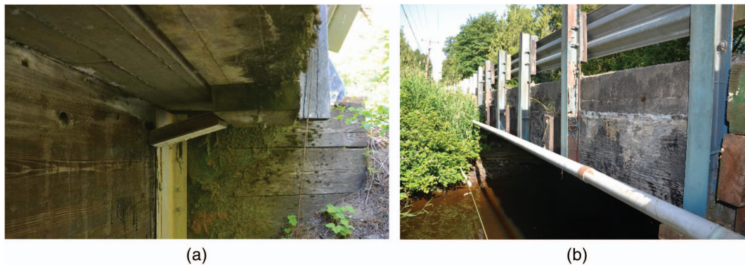
Fig. 11. (Color) (a) Good; and (b) bad examples of concrete overhanging. (Images by Alfredo M. P. G. Dias.)
