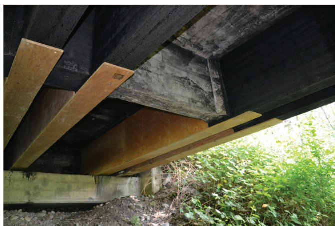
Fig. 13. (Color) Fire damage in the timber members of a TCC bridge (treated plywood was added to reduce the fire damage potential). (Image by Alfredo M. P. G. Dias.)
