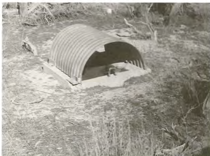
FIGURE 7. A satellite water source for small animals served by a buried pipeline. Such "birdbaths" provide reliable drinking water for wildlife even when the main pipeline is not active if associated storage tanks are installed.
