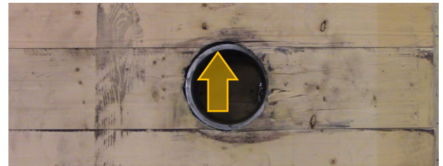
(a) Hole elongation around steel bushing
