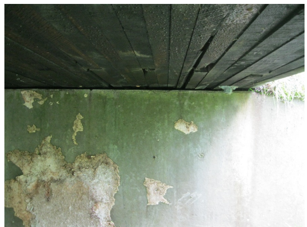
Figure 12 Hoffman Run deck uplift at corner bearing
