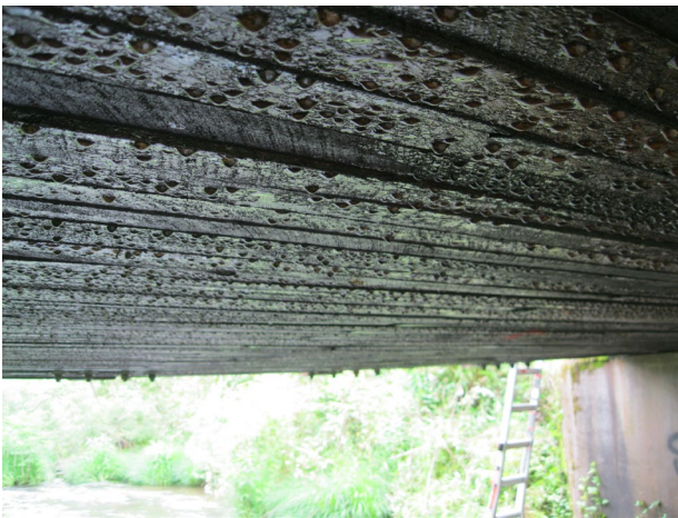
Figure 14 Hoffman Run underside water accumulation
