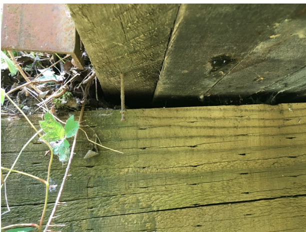
Figure 10 Hibbsville deck uplift at corner bearing
