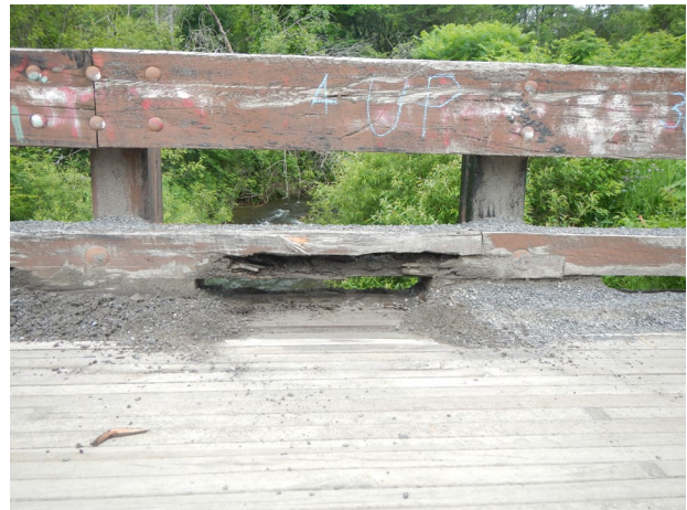
Figure 16 Hoffman Run debris accumulation leading to significant decay of curb members.
