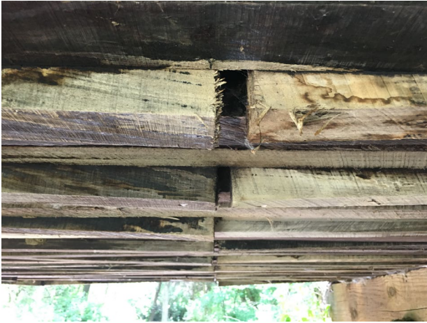
Figure 8 Hibbsville gapping at lamination butt joints
